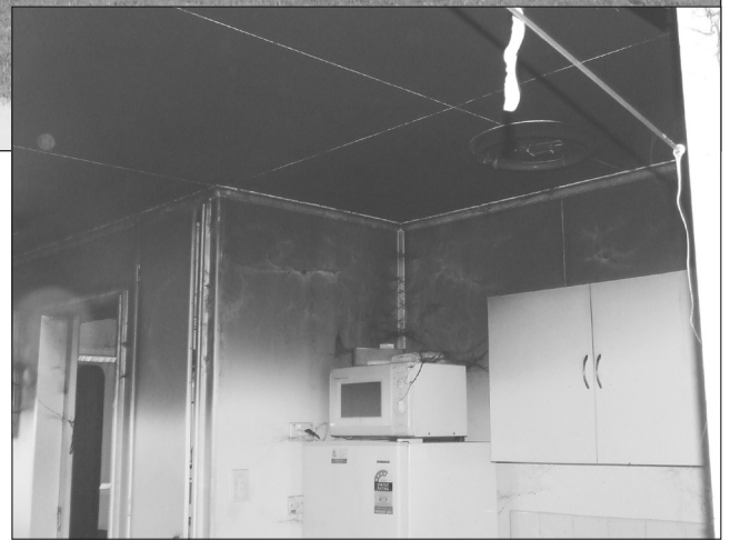
RIGHT: Smoke and heat caused extensive damage to the interior of the Unit.
