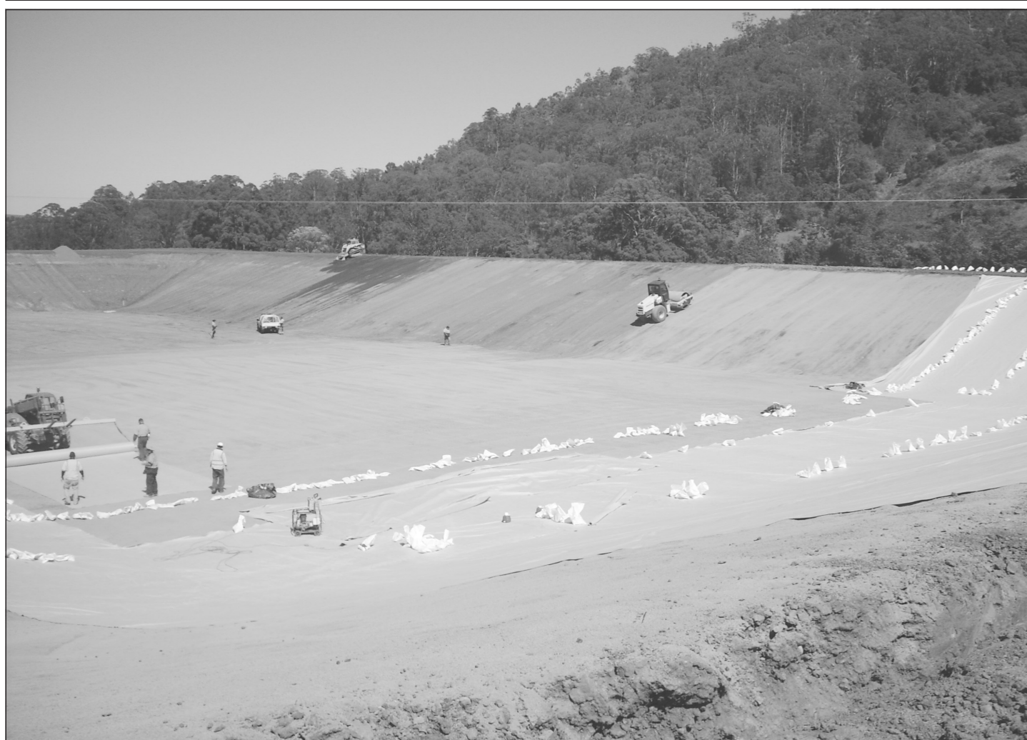
Picture taken of the new Killarney off-stream storage facility last wednesday, 20th January, at about 9.30am: Southern Downs workforce preparing the Off Stream Storage. Final trimming and placing of a crusher dust layer was done. Darling Downs Tarpaulins installed a geofabric layer prior to installing the HDPE lining. About 20000 litres of water a day is flowing through the underdrains installed under the HDPE Lining. Photo © Jim Llewellyn
