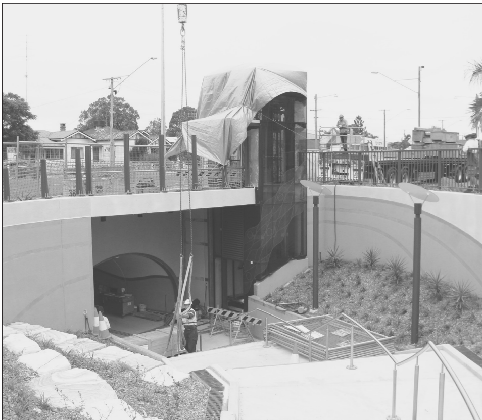
The crane unloading the lift equipment last week at the Underpass construction site.
