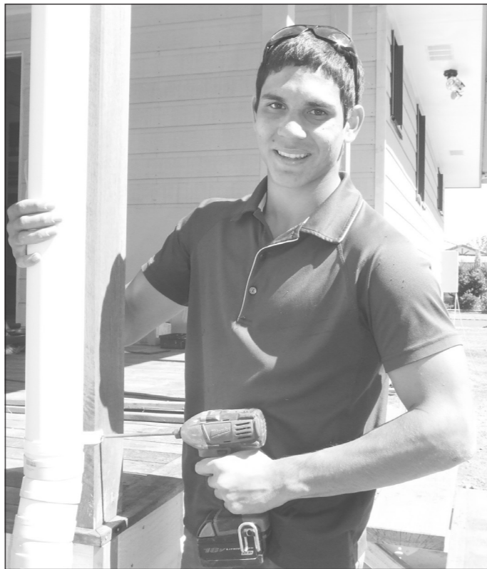
Brodie Frizzell secures a downpipe on a new home being constructed, while undertaking work experience with Kev Harrison of Allora's Harrison Plumbing.
