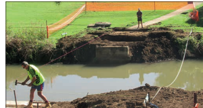
Work is well underway on replacing the old wooden bridge near the 9th green at the Allora Golf Course.
