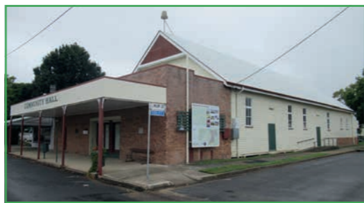
approved repairs to the Allora Community Hall, which has been out of action since structural problems were identified early in 2022.
