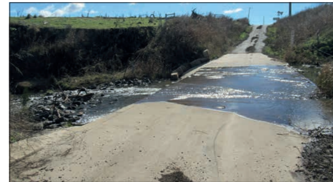
Merivale St After flooding and out of action
