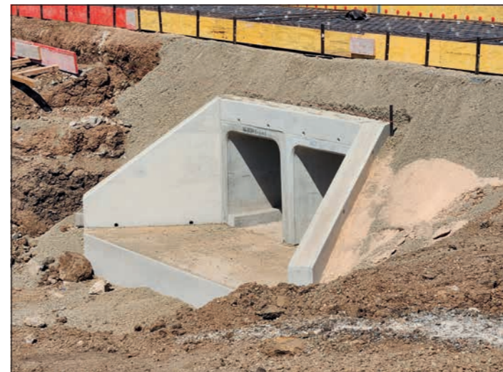
Photo Dave Burns
