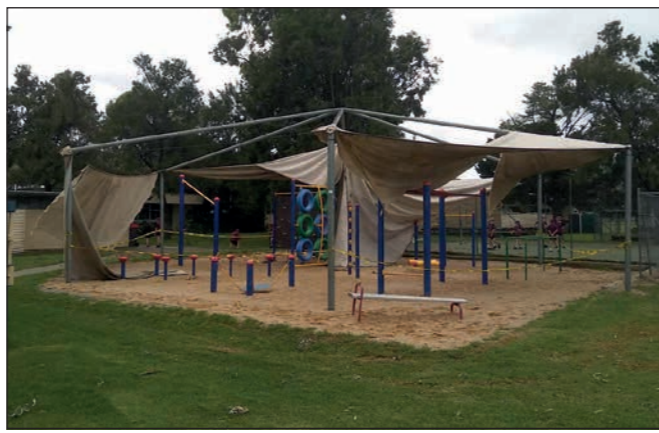
The shade cloth over playground equipment at Allora P-10 State School was shredded during the storm.
