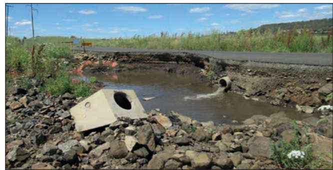
Flood damaged culvert in Merivale Street Allora.
