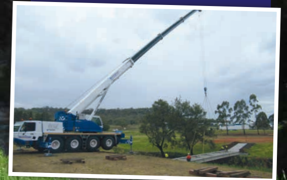
Below The Maher-Rickert Bridge being craned into place. The new bridge now allows golfers to cross the Dalrymple Creek more safely when playing the 9th and 18th hole. The old weir crossing is no longer being used.
