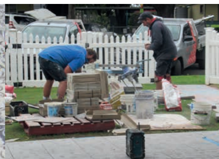
Tony Morris Tiling seen here laying tiles in the Sports Club's alfresco area.
