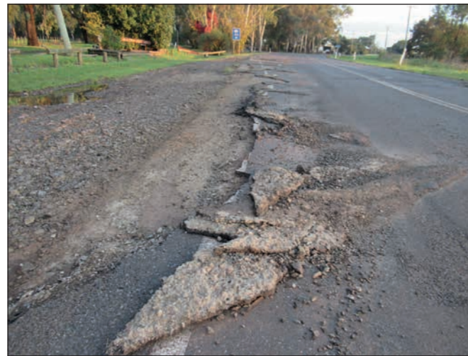
Flood damage to the surface of Allora Drive near the Park.
