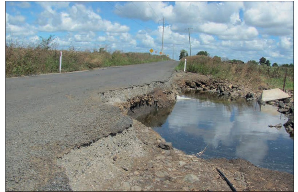
ABOVE: Flood damage to Merivale Street.
