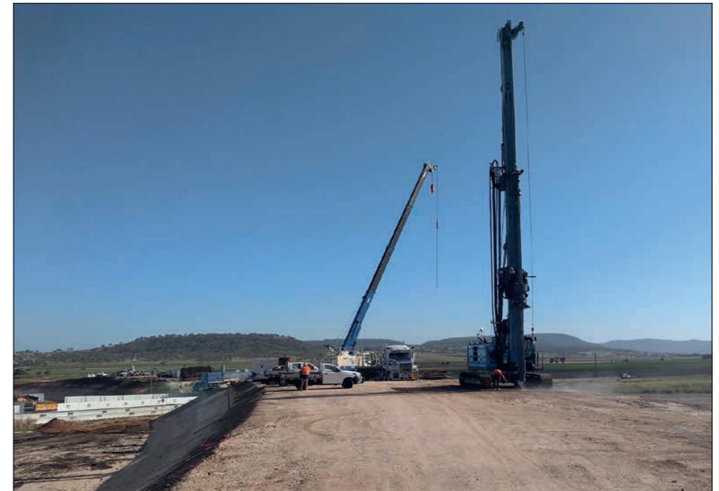
The drill rig was used to bore down 26 metres to install the bridge foundation piles for the overpass at Eight Mile intersection. The crane in the background was used to lower in reinforcing steel to the abutment piles. (Photo courtesy Department of Transport and Main Roads)
