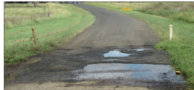
In our district there's quite a few roads with damaged surfaces due to the wet weather. This crossing near Rix Road on the Hendon-Mt Marshall Road is a good example with large pot holes.
