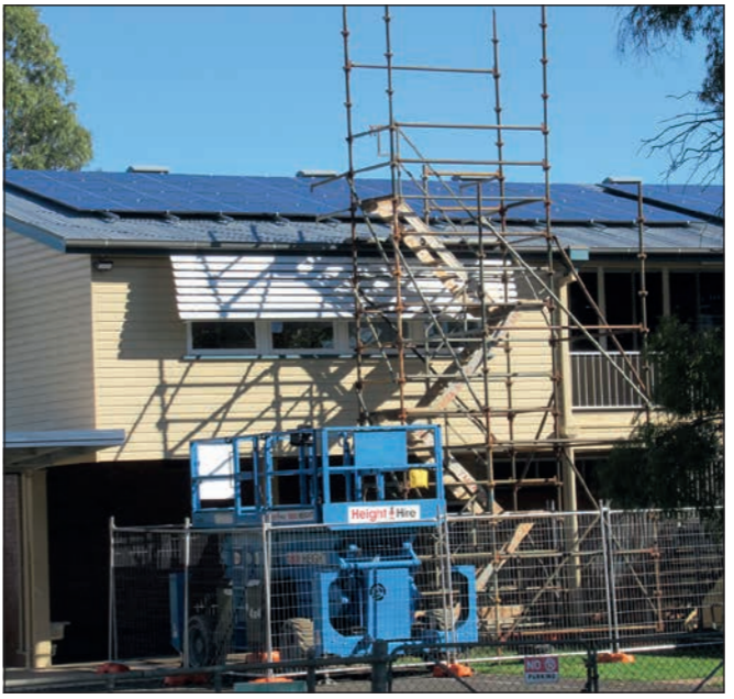
Work underway as part of the Advancing Clean Energy Schools Program with solar panels being installed.
