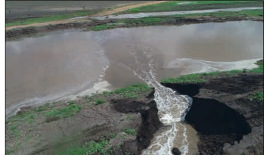
As reported elsewhere this is NOT the Quarry Dam but the Farm Irrigation Dam on Bolzan's property.
