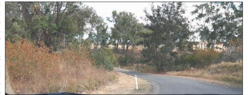
Before: Approach from east shows vegetation masking the view of the western approach.
