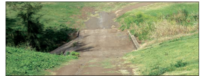
Golfers will no longer use this old weir crossing over Dalrymple Creek after the construction of the new bridge.
