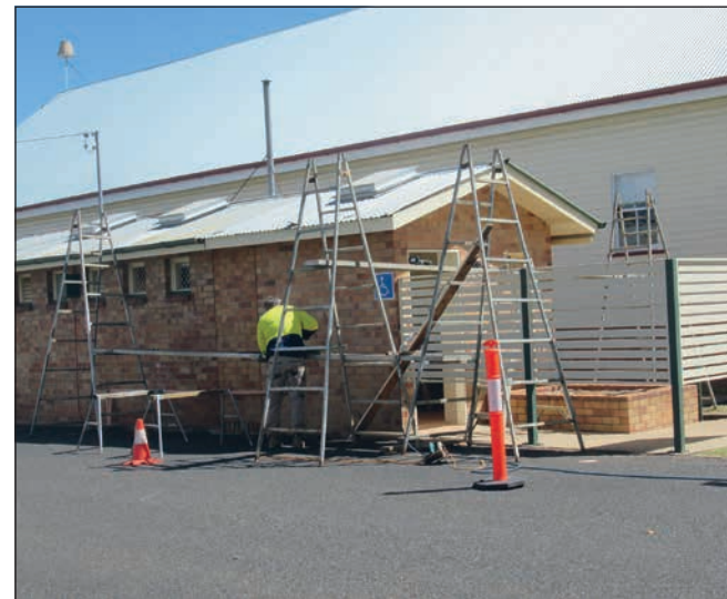
Repairs being carried out to the surrounds of our Public Toilets in Muir Street after a driver reversed into them. Must have been in a hurry!
