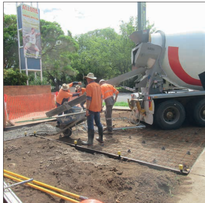
Southern Downs Regional Council workers are busy laying cement and clearing the area in readiness for the erection of the Laura Geitz statue to be unveiled on Saturday 21st March.
