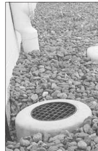
A standard modern Overflow Relief Gully.
