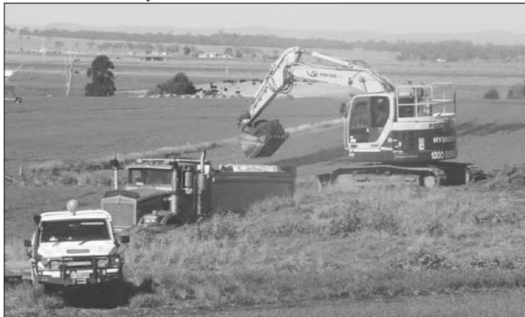
Excavator levelling the mullock heaps at the old Allora coal mine, off Hillside Road.
