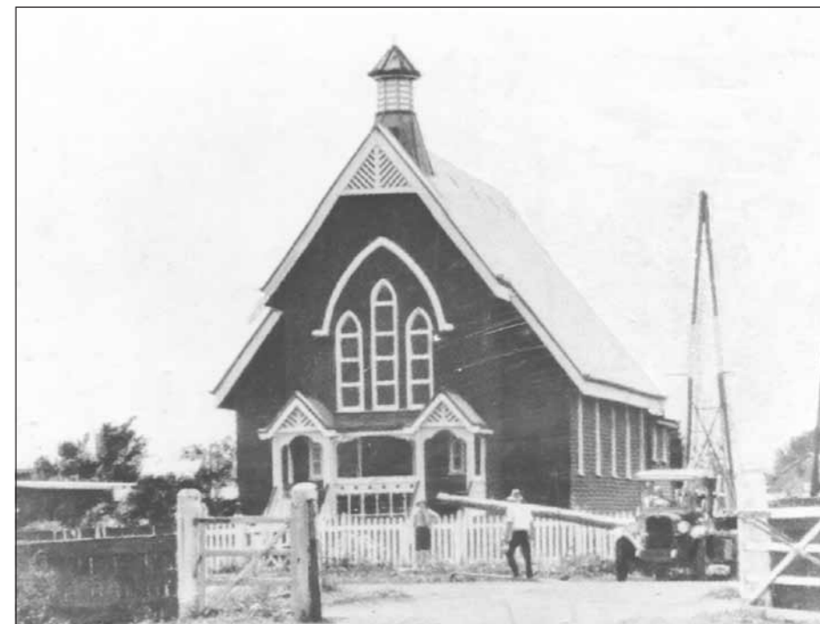
Truck and derrick erecting power poles next to St. Andrew's Church in 1932.
