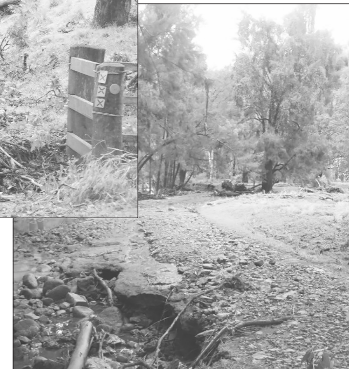
Road damage between Mill and Rock crossings.
