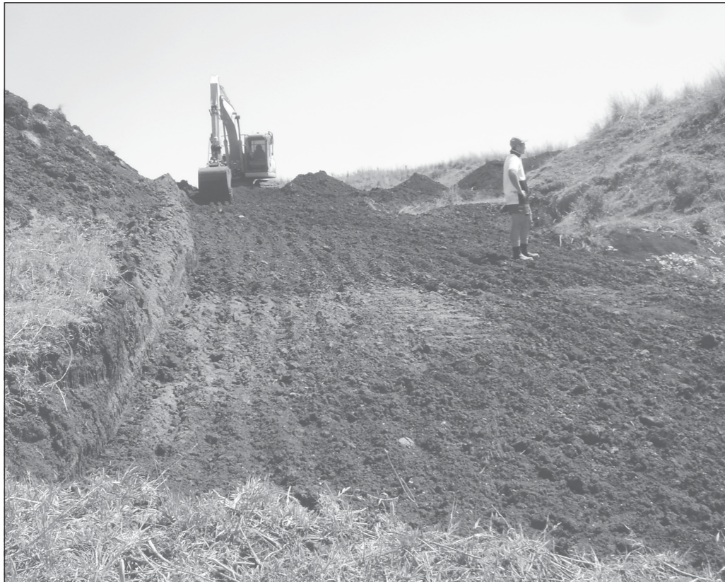
BYE GULLY: MRP Earthmoving flatten and reshape the severely eroded gully along Dalrymple Creek Road in the final gully stabilisation job as part of Condamine Alliance's flood recovery program.
