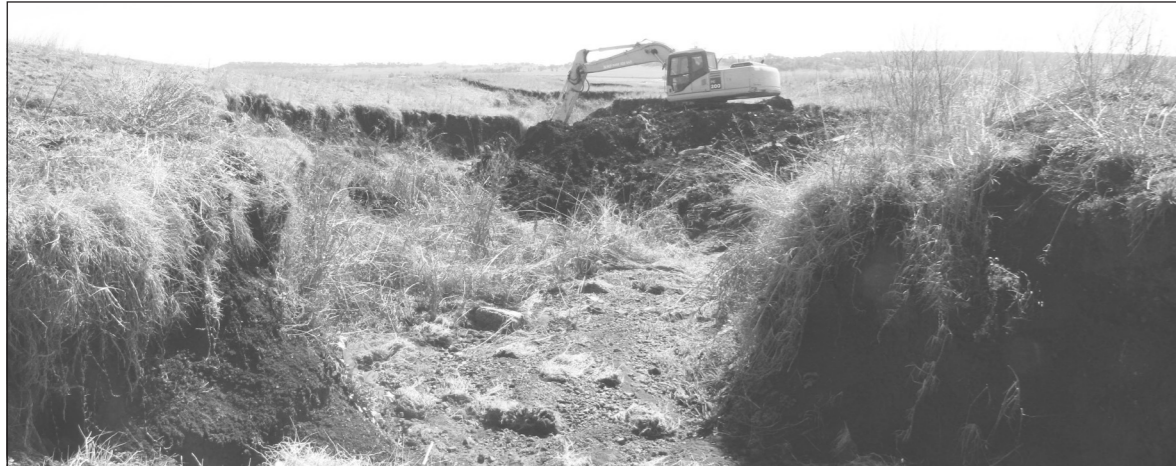
LEFT: BEFORE - Damaged gully at Greenmount site.
