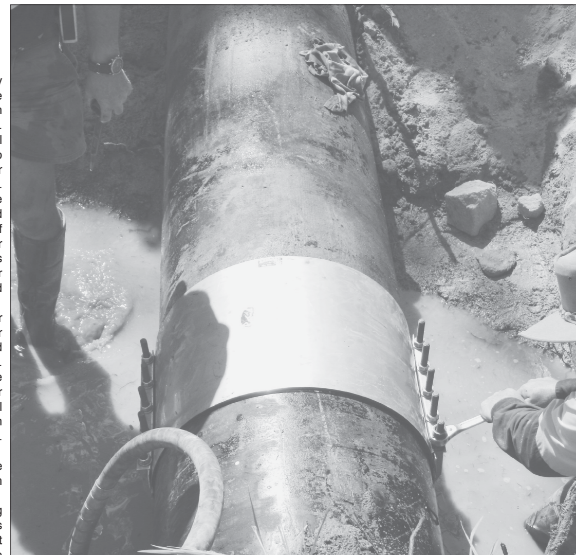
Repairs to the 600mm wide water main delivering water from Leslie Dam to Warwick.
