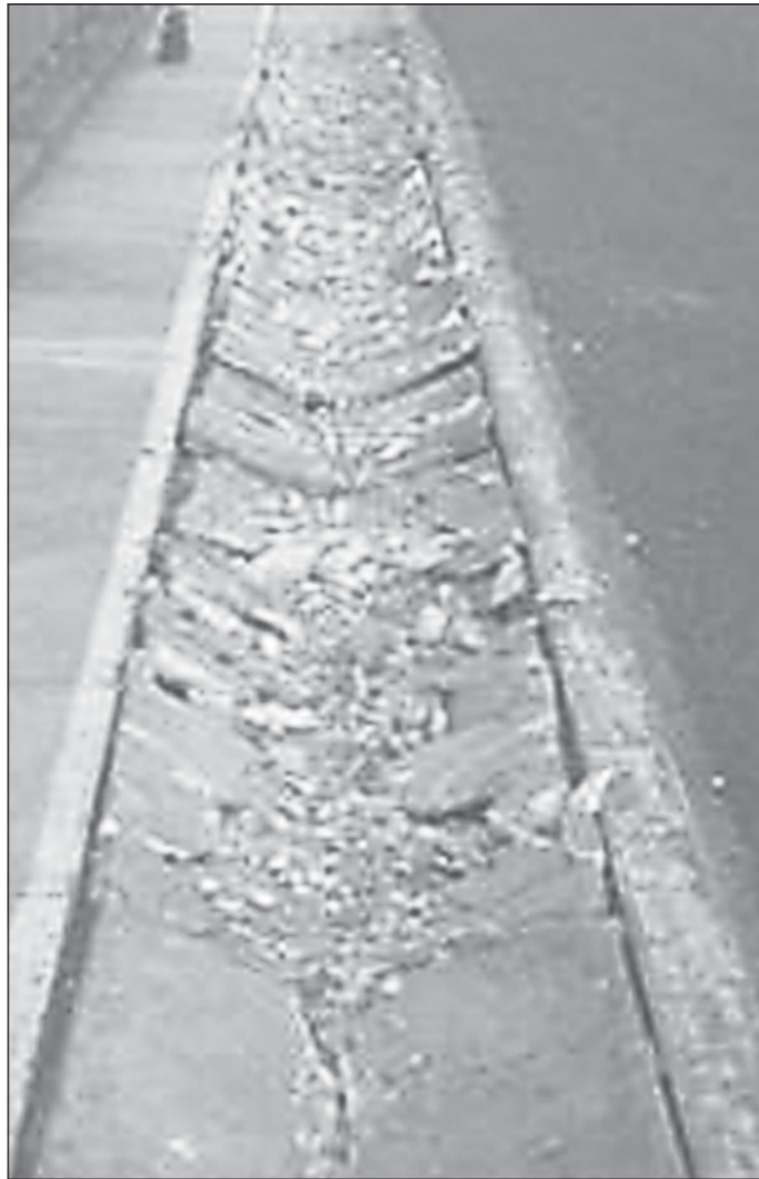
Heavy vehicle damage along McCahons Bridge in Warwick.
