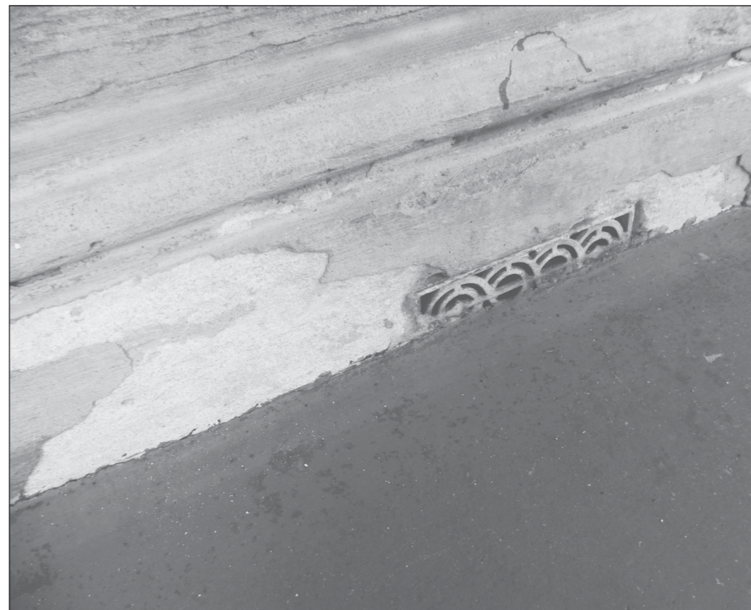
An example of a ventilation outlet that has been partially covered by raised levels. Initially there was a step up to the Town Hall from the street level. On either side of this ventilation outlet the stonework has been worn away. The restoration will see a sandstone process used to make blocks like these look as good as new.
