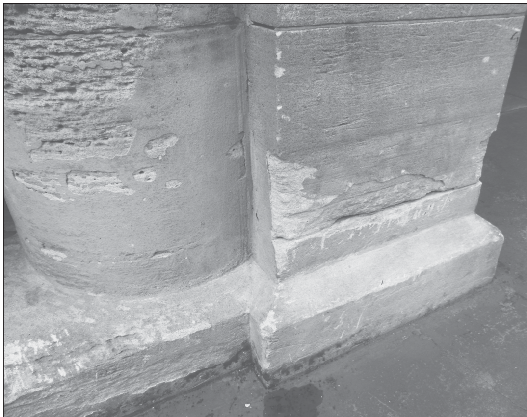
Queensland Heritage Masonry will attempt to repair the columns to the original condition, however, the columns are more difficult to restore than the flat stonework.
